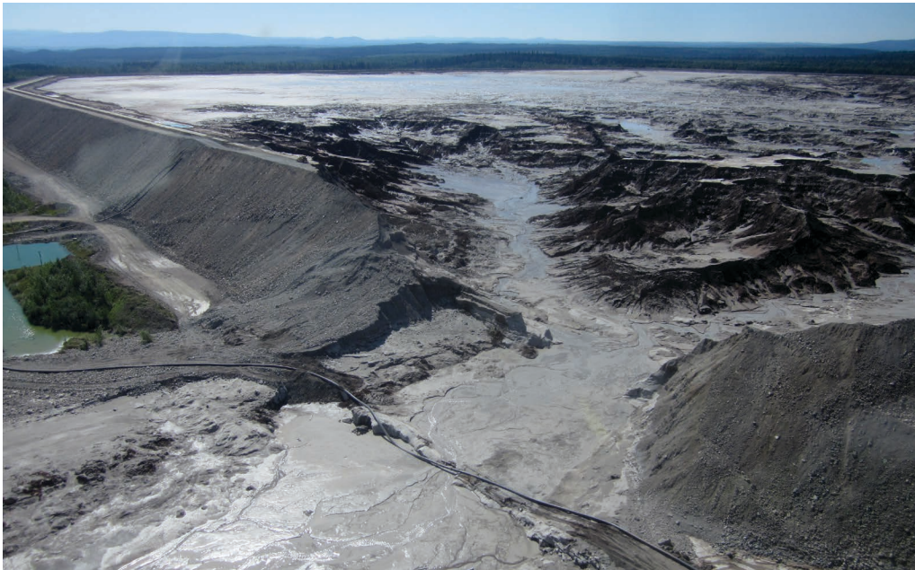
COLLAPSED MT. POLLEY TAILINGS DAM WALL, FOUR DAYS AFTER THE BREACH. PHOTO: RICHARD HOLMES.
